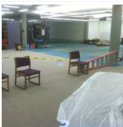
The aftermath of the Zimmerman Library flood as a result of a torrential downpour that hit the University-area in August 2014.
